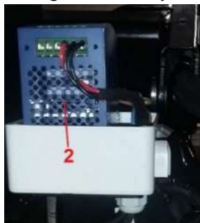
2 = Converter 230V AC/ 12V DC
